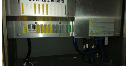
(b) Inside the controller we can see various connectors and cables exposed. The left side includes I/O and safety, whereas the right one leads to the main computer.
