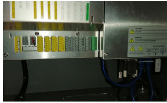
B) Inside the controller we learn about connectors and cables, which are exposed. The left side includes I/O and safety, whereas the right one leads to the main computer.
